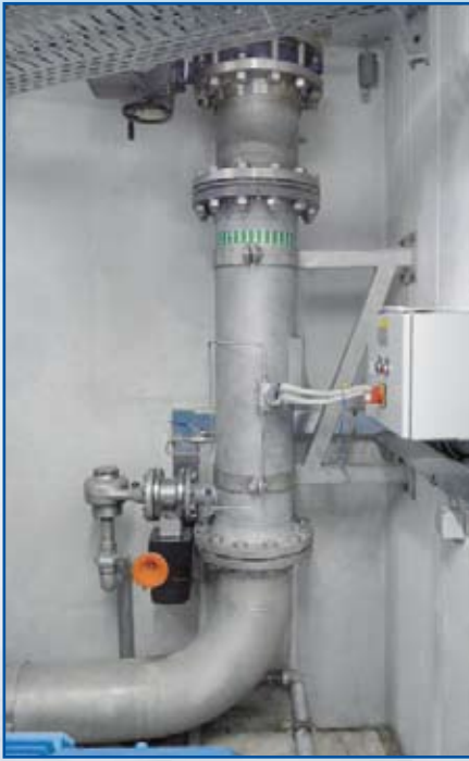
Fig. 8 sea water filtration for snow making system
