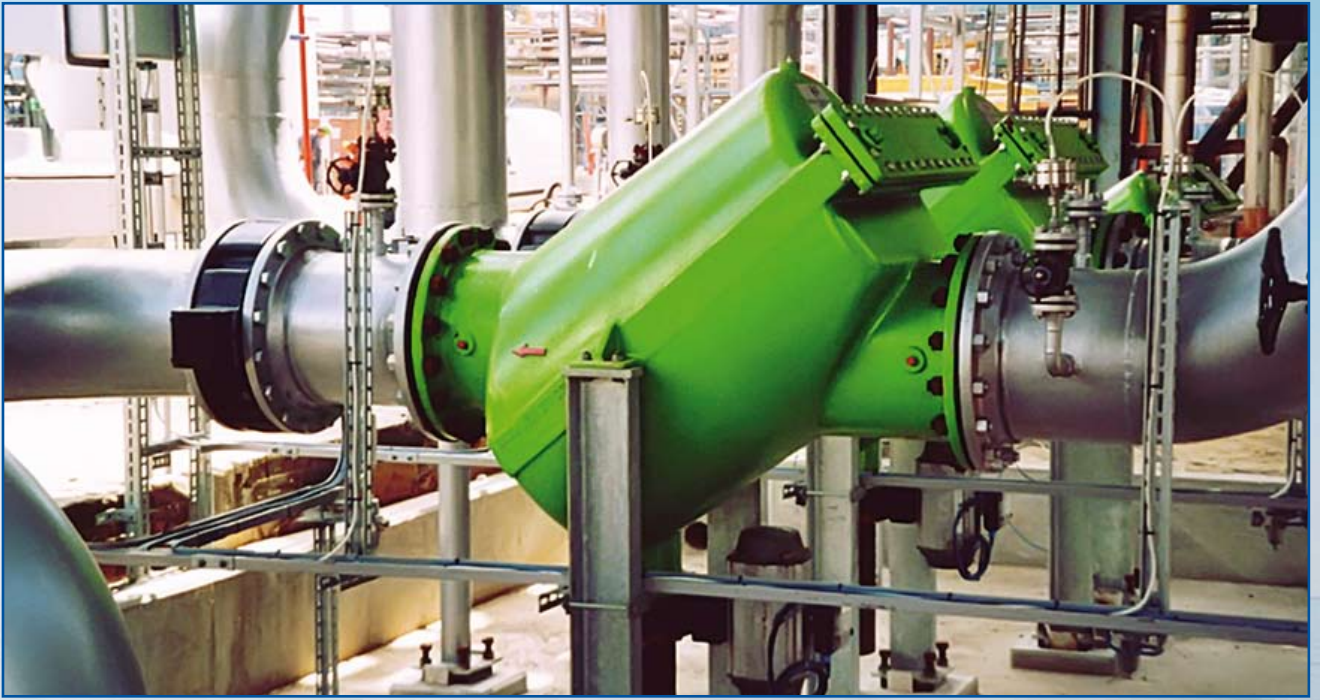
Fig. 09 sea water cooling water filtration in a refinery
