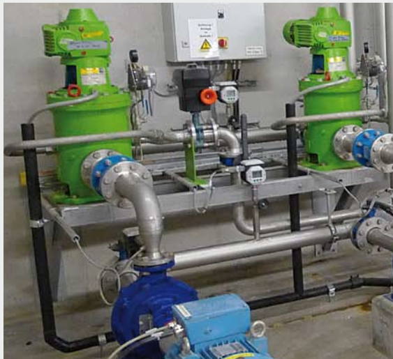
Fig. 4 sealing water filtration in power plant
