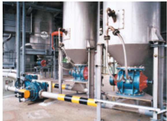
Product feed from silo via rotary valve.
