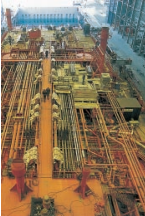
AG AIR DRYER in action to provide dry conditions for surface treatment.
